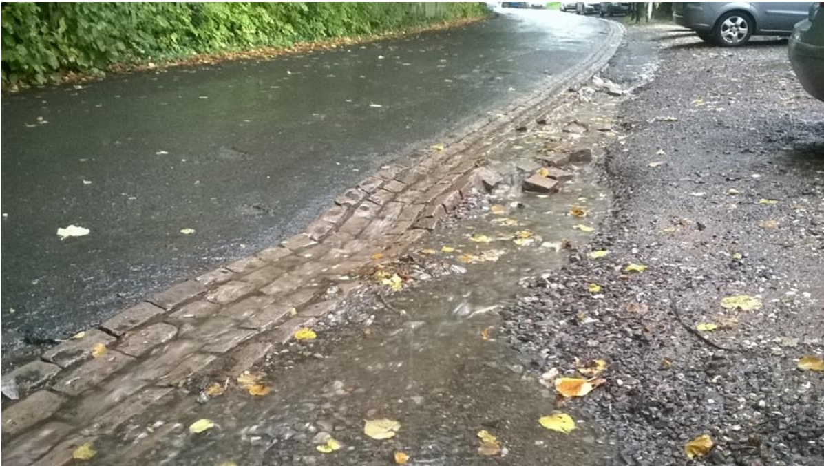
The Warren. The road gutter nearest to the wall is being increasingly eroded by heavy rain creating a river effect. This, in turn is eroding the ground between the wall and the road.
