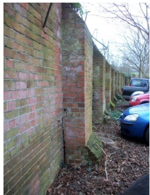
Brick boundary wall to Caversham Court Allotments on The Warren in disrepair
